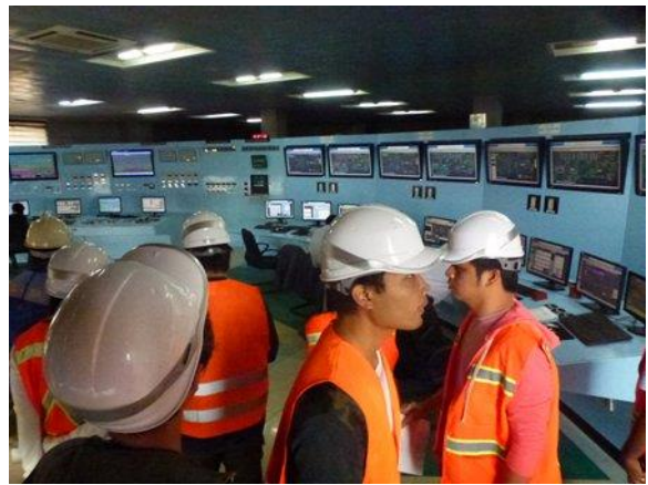
In the control center
